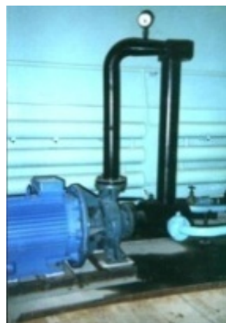
Fig. 5. Vortex hydraulic heat generating plant
